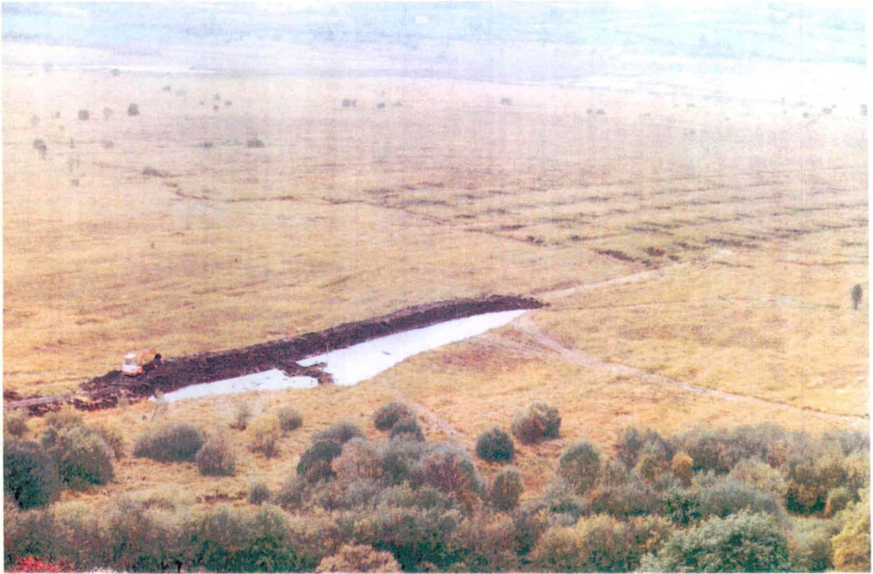
Construction of a bund around old peat cuttings on the SE bog at Cors Caron (Dyfed). The lines of dams across ditches on the remaining 'dome' of the bog can also be seen. [Photo: J.E. Davis]. [see also Plate 5.6]
